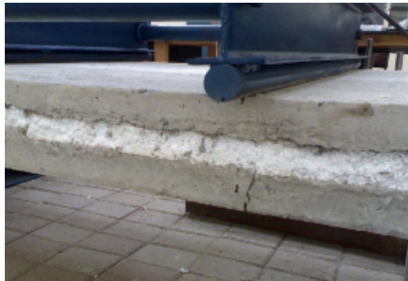
Figure 5: Cracking Pattern in two Layer Panel
