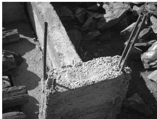
Figure 10: Steel Bars In Column With Uneven Cover And Improper Placement
