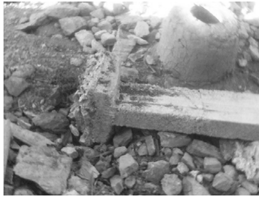
Figure 8: Inadequate footing of a slender column
