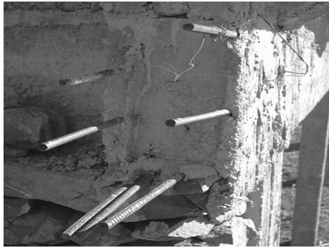
Figure 11: Improperly Placed Steels Bars In A Beam
