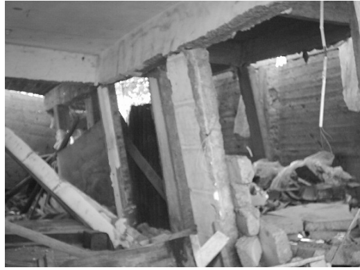
Figure 2: Concrete Frame Exhibiting Large Sway
