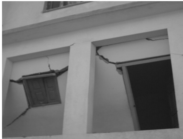
Figure 12: Un-Reinforced Concrete Wall Panels Collapsed Due To Earthquake
