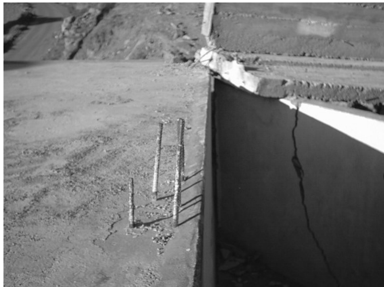
Figure 5: Insufficient Dowels Lengths Left For Extension Of Mosque In Pambara Village
