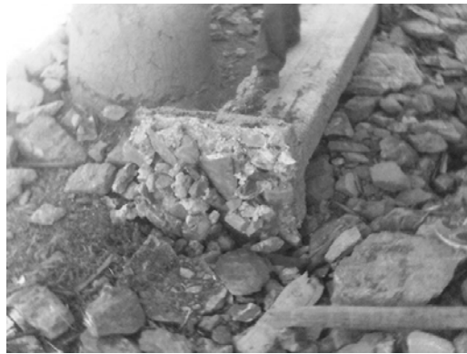
Figure 9: Inadequate column footing
