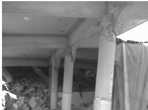
Figure 3: Joint Failures Of Balakot Jamia Mosque
