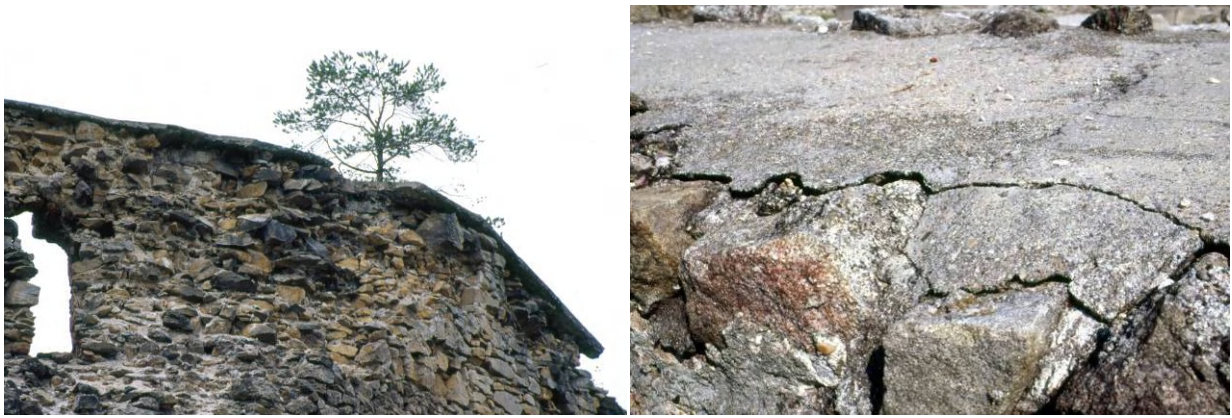
Figures 3, 4: An interesting example of conservation of the castle of Liptovský Hrádok (Slovakia) sometimes during the 30-ties (left). A layer of concrete was simply placed over the wall copings, which did not protected the wall below against the rainwater very effectively, but it has anyway saved the shape of the ruin for the following 80 years. Right a newly placed concrete (80-ties) over o top of a roman castle ruin in Gerulata (Bratislava, Slovakia) – cracks in concrete are already visible, which allow rainwater to penetrate the original masonry and the concrete cover is already separated from the original by a huge sheet breakaway.
