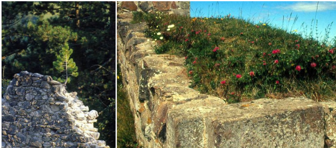
Figures 15, 16: Unwanted vegetation – a small tree on the walls of the Sklabiňa Castle in Slovakia, which should be immediately removed, and a nicely planted grass and flowers cover on the top of a wall of the Brahehus ruin in Sweden – even such a type of the cover has some limits of its technical life, given by relative low erosion resistance of the sides of the “flower-pot”.
