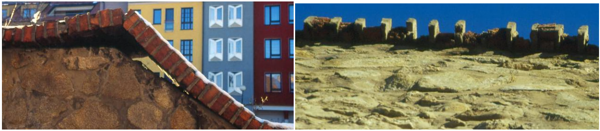
Figures 10, 11: Use of materials with very different physical characteristics in comparing to the original ones (both are examples of the city walls in Bratislava, Slovakia) – on the left the dilatibility of the wall coping made from brick on cement mortar is much different to that one of the stone masonry, on the right the use of materials with very different erosion resistance (very hard cement mortars combined with weak bricks) has lead to continuous degradation of the brick part of the coping, where only the cement mortar in joints could resist the erosion – very funny appearance of the wall coping was reached (unplanned).
